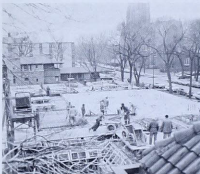
McGiffert House under construction (looking west, Robie House and Rockefeller Chapel in background.)
